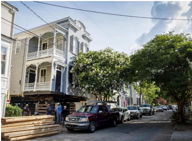
Recurring flooding is compelling some to elevate their houses in Charleston. Raising a historic home can cost hundreds of thousands of dollars. Matthew Fortner/Staff
