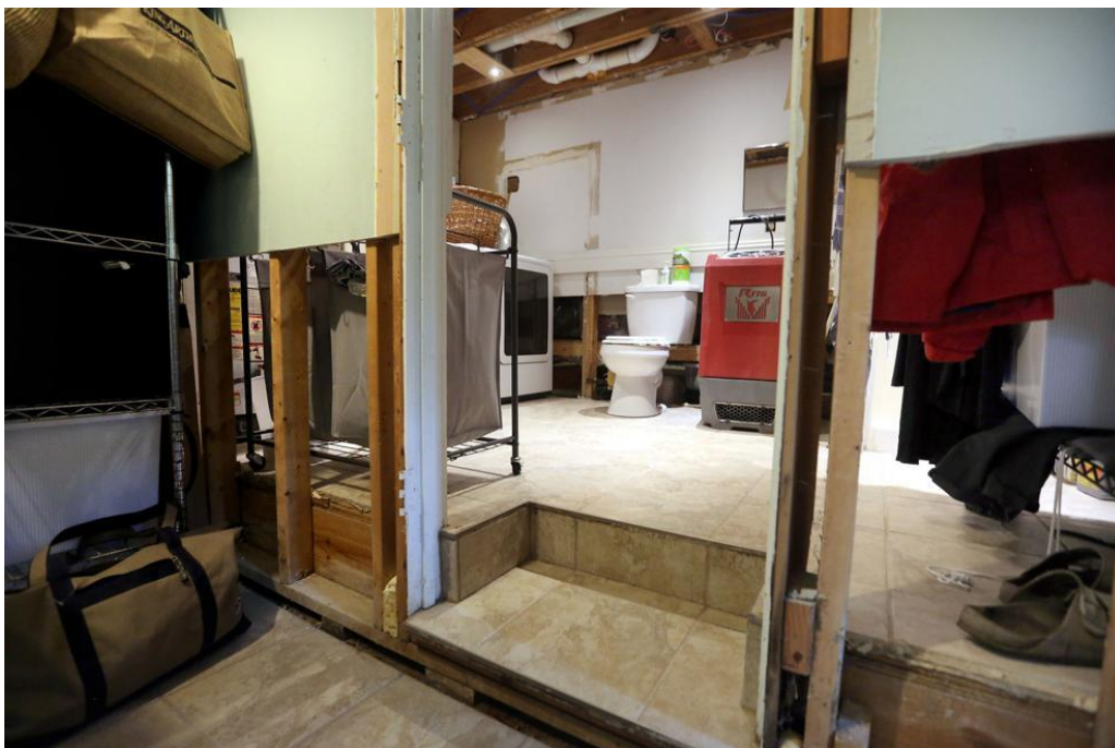
Flood damage to the first floor of Kurt Oberle's Seaward Drive home on James Island. Brad Nettles/Staff
