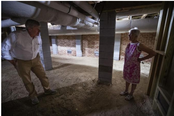
Buz Morris, president of Morris Construction, and Margaret Perry stand under her house on Council Street on Thursday, July 18, 2019. Laurent Petracca/Staff
